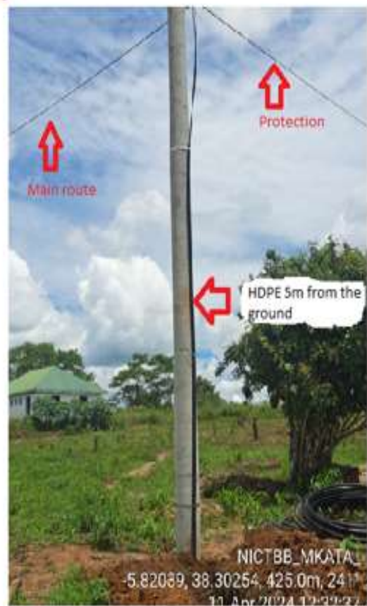
NICTBB office terminal pole
